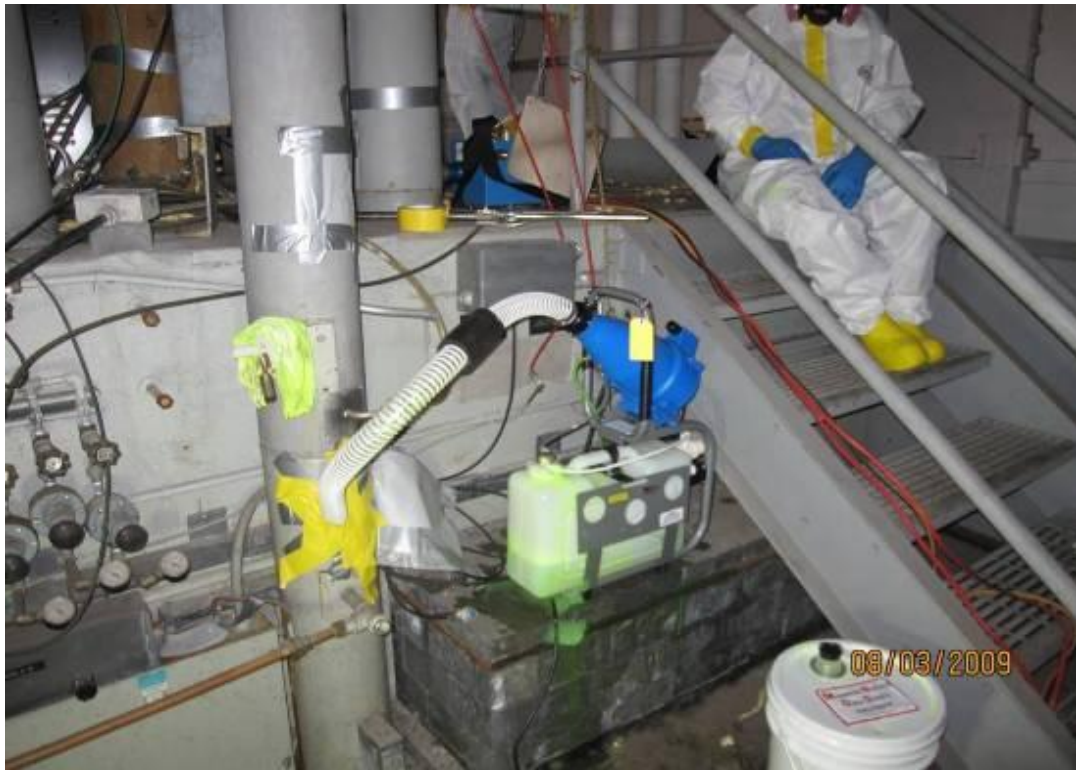
Delivering CC Wet into the Cell Bank 2 via the cell ventilation duct.
